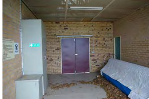
10) Main entry & first aid 'area' in large cup board – unacceptable. Exposed in main entry
