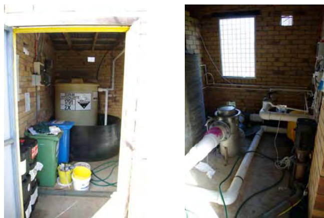
27) Pool Filtration plant – “Hypo- tank’ storage unit with additional chemical store. 28) Filter and main pool pump.
