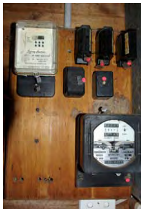
33) Switch board / meter board – may contain asbestos, due to its age and condition.
