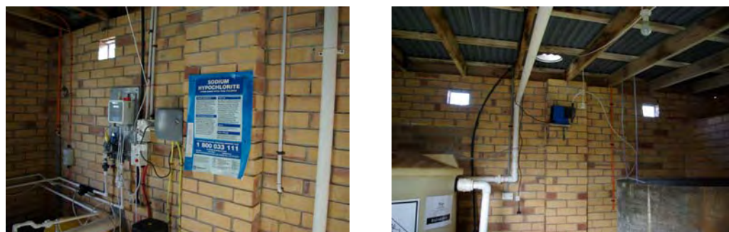
29) Current dosing system 30) Chlorine pump – to high.
