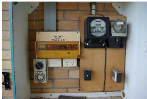
40) Backing to switchboard may contain asbestos.
