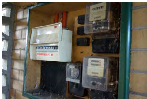
42) Main switch board and meter board backing may contain asbestos.
