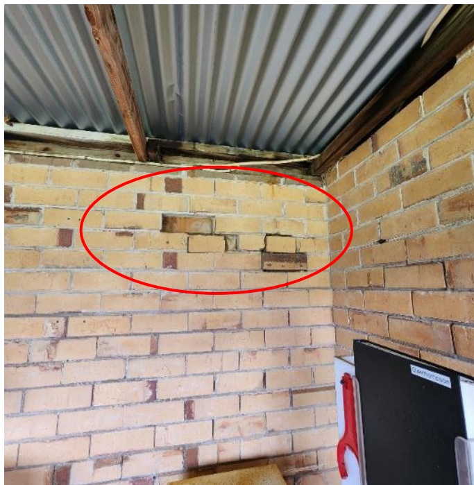
Image 40: WTP dislodged bricks in north wall
