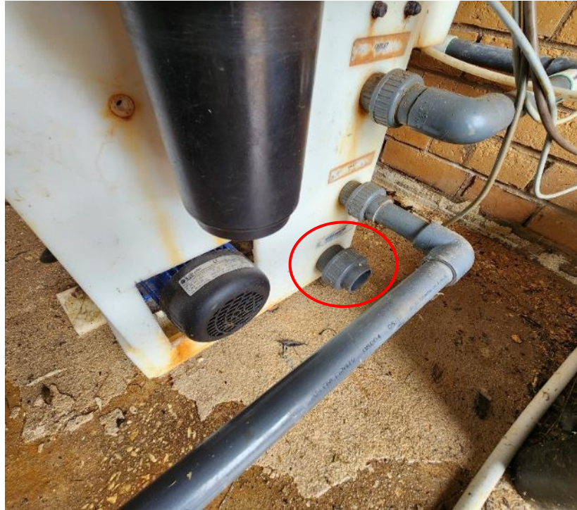
Image 29: Over-flow from cal-hypo unit discharges to floor
