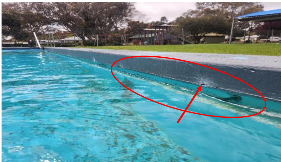
Image 11: Main pool, Shallow end hob on water side. Cracks starting due to reinforcement corrosion.
