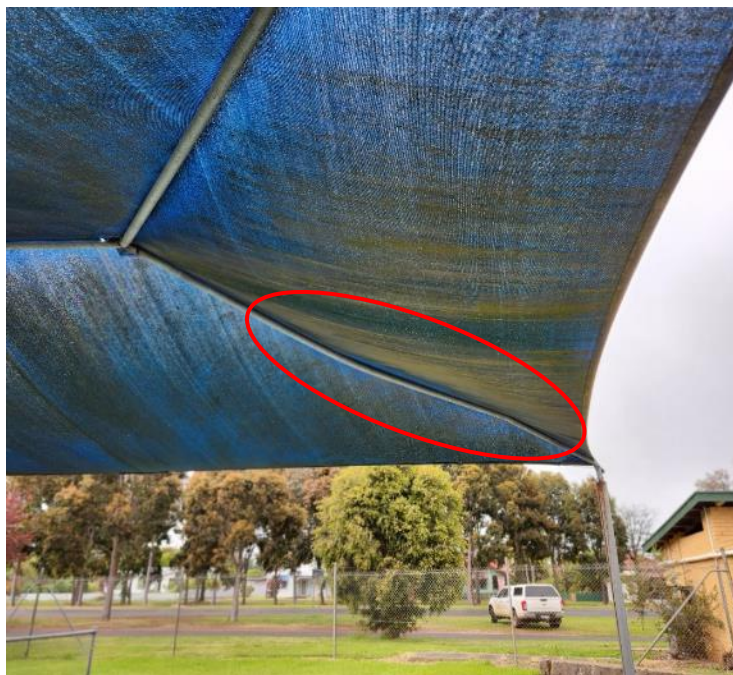
Image 42: Toddler's pool, shade structure. Bent (technically failed) structural support tube.
