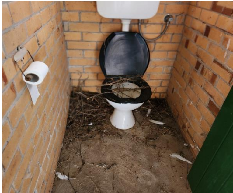
Image 35: Changeroom (male) – debris from wind, and bird entry
