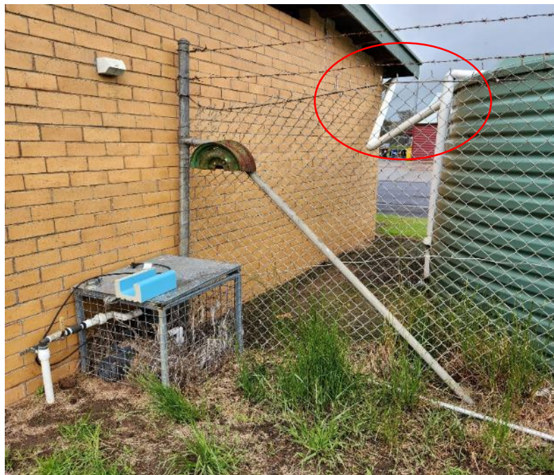
Image 44: Rainwater recycle pump. Note dislodged infill pipe.
