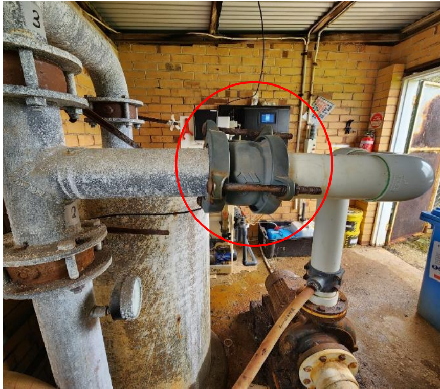
Image 31: Unsupported Gibault joint in discharge pipework
