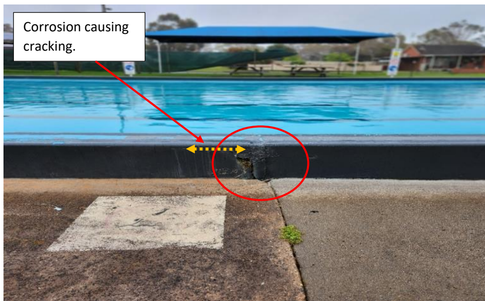
Image 13: Main pool. 'Bulging' expansion joint, east side. Hob cracking due to reinforcement corrosion.
