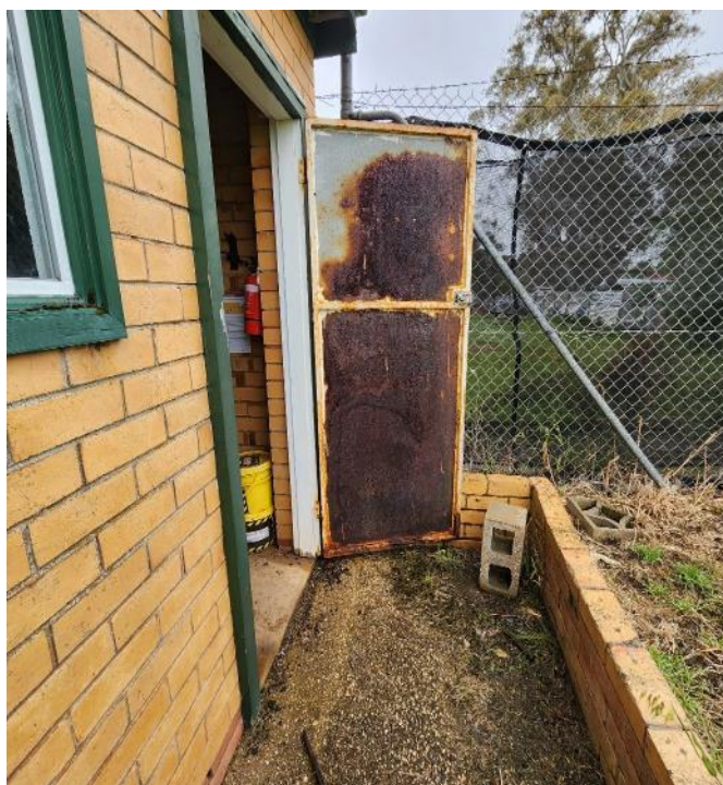
Image 41: WTP door is badly corroded.
