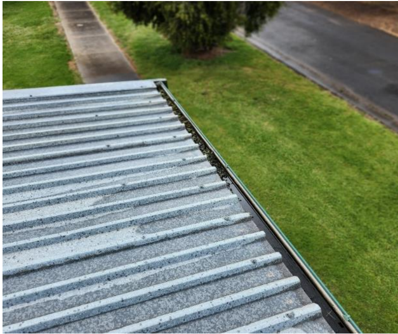
Image 37: Changeroom roof- blocked gutters holding water.
