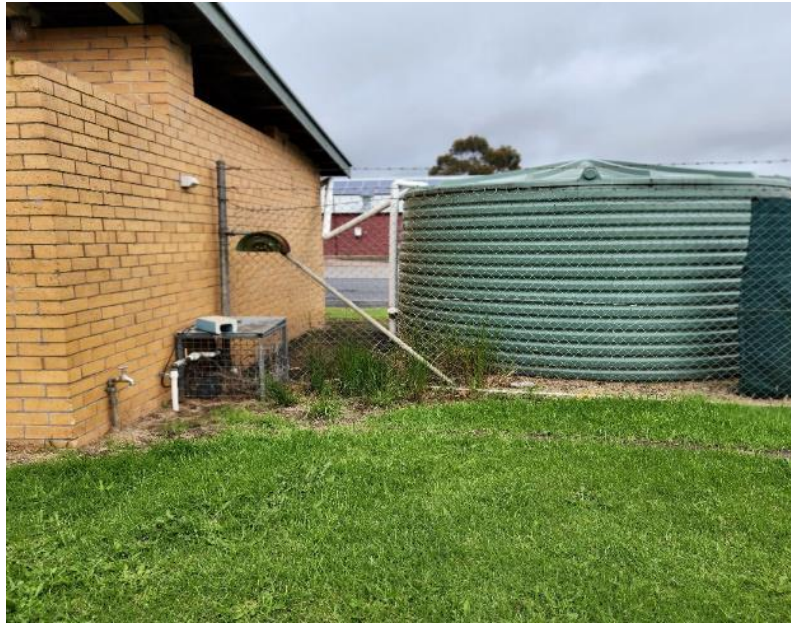
Image 43: Rainwater harvest tanks and pump
