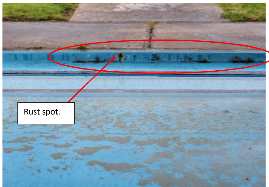
Image 21: Toddler's Pool. Crack in floor/wall through centre of pool, west side
