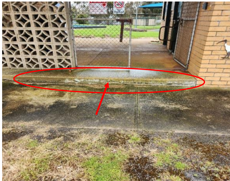
Image 38: Entry to facility. Long crack along front of slab edge due to reinforcement corrosion.
