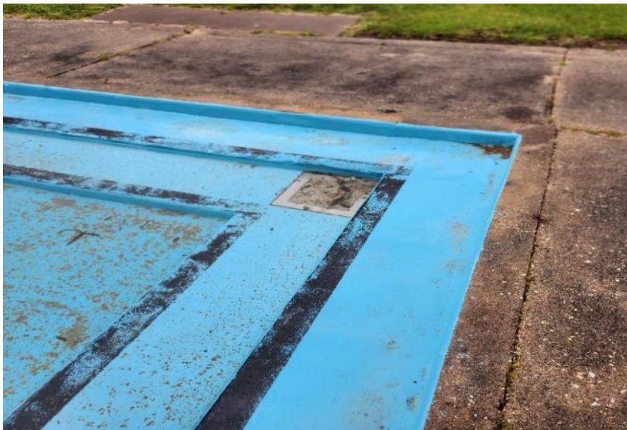
Image 19: Toddler's pool. Soiled Water outlet grate, SW corner
