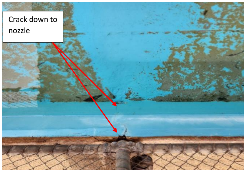
Image 20: Toddler's Pool. Crack in floor/wall through centre of pool, east side. Looking down vertically.
