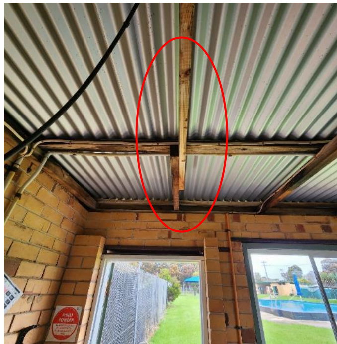
Image 39: WTP new roofing iron but with inadequately spliced rafter
